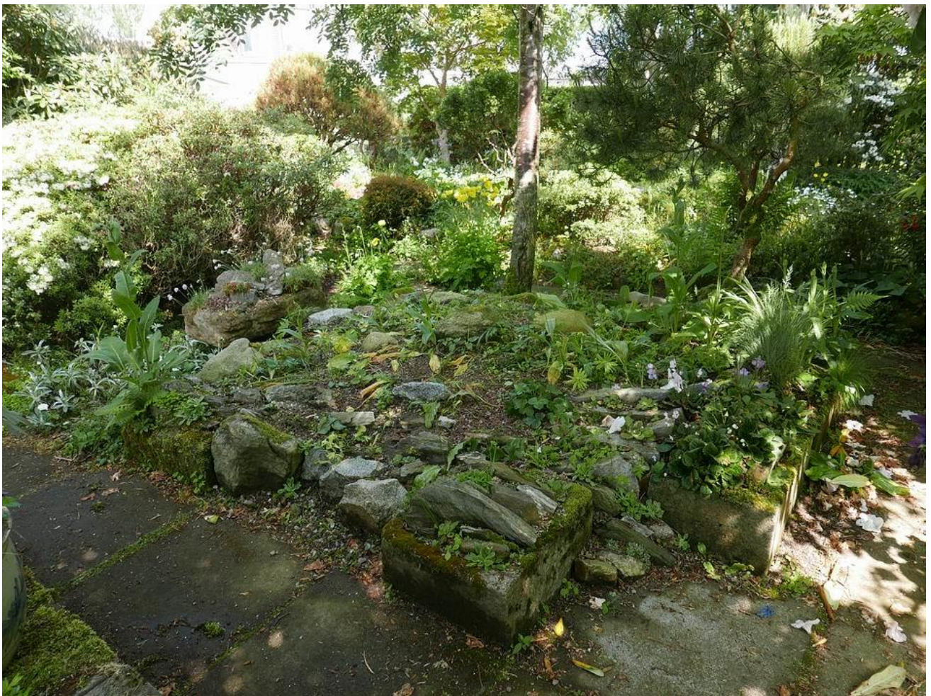
With the construction work behind me I can now concentrate on the planting which links nicely into my desire to cut back on the number of bulbs we grow in pots because I was going to release many of those special plants from pots and plant them here in this new bed.
